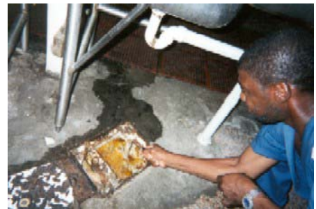
Grease trap at Young Island Resort, St. Vincent
