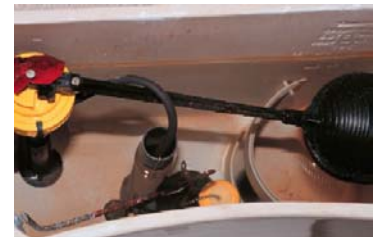
A toilet dam installed at Treasure Beach Hotel.
