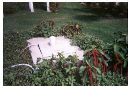
Oualie Beach Hotel, St. Kitts: Gray water treatment system, designed in Nevis, and masked by vegetation. Water from the laundry and other areas is sent through this area and subsequently used for the gardens.
