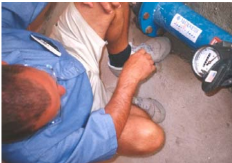
A water meter at Club Dominicus Palace, Dominican Republic
