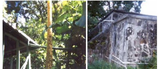
Above left: Rainwater guttering at Papillote Wilderness Retreat, Dominica.
